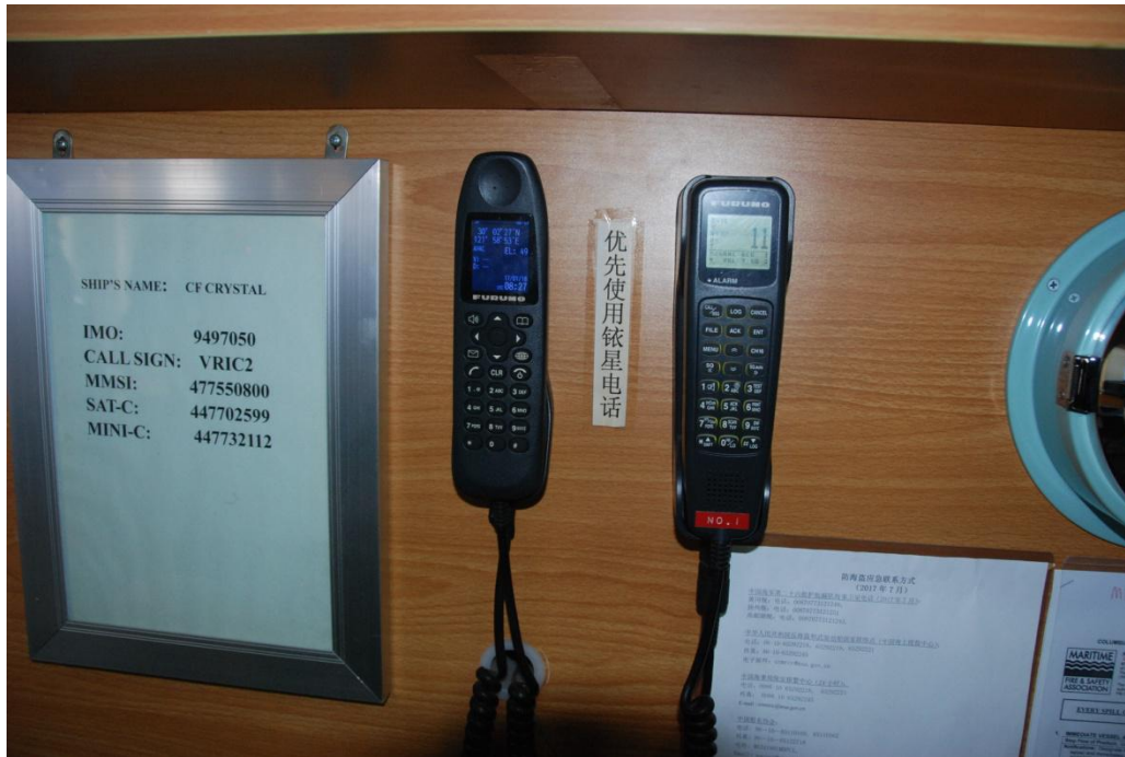
VHF and Sat Phone (Radio Room)
