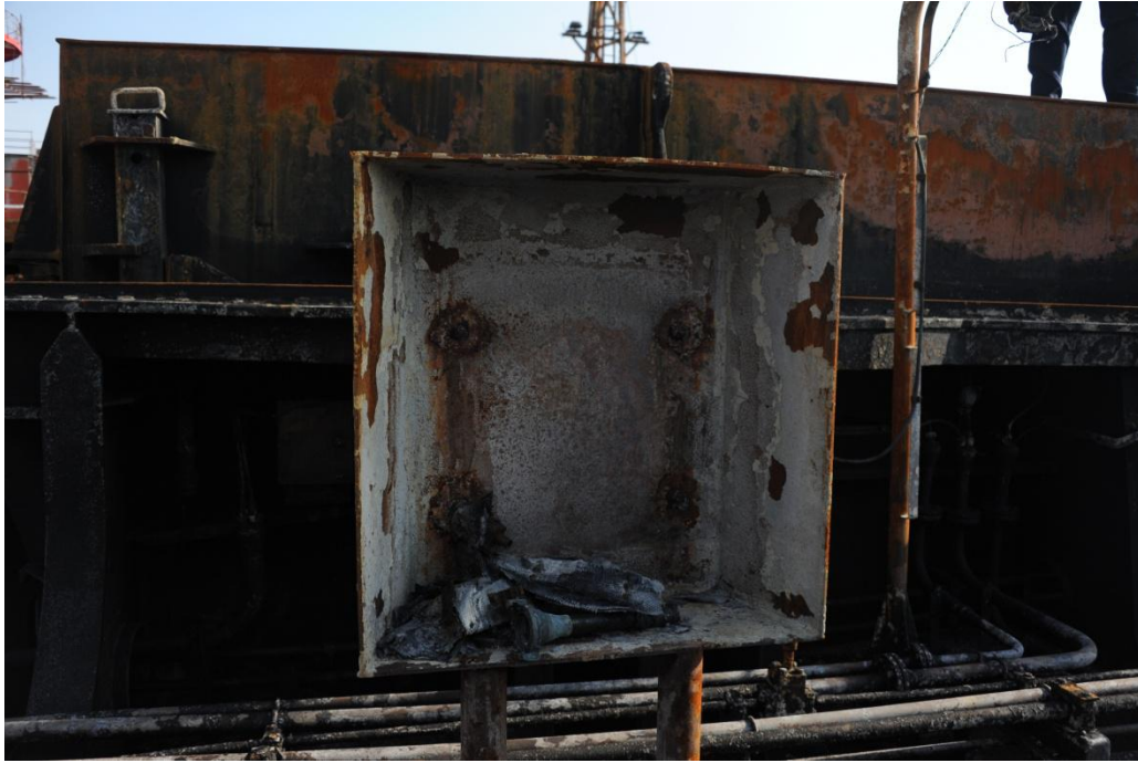
Fire Box Debris
