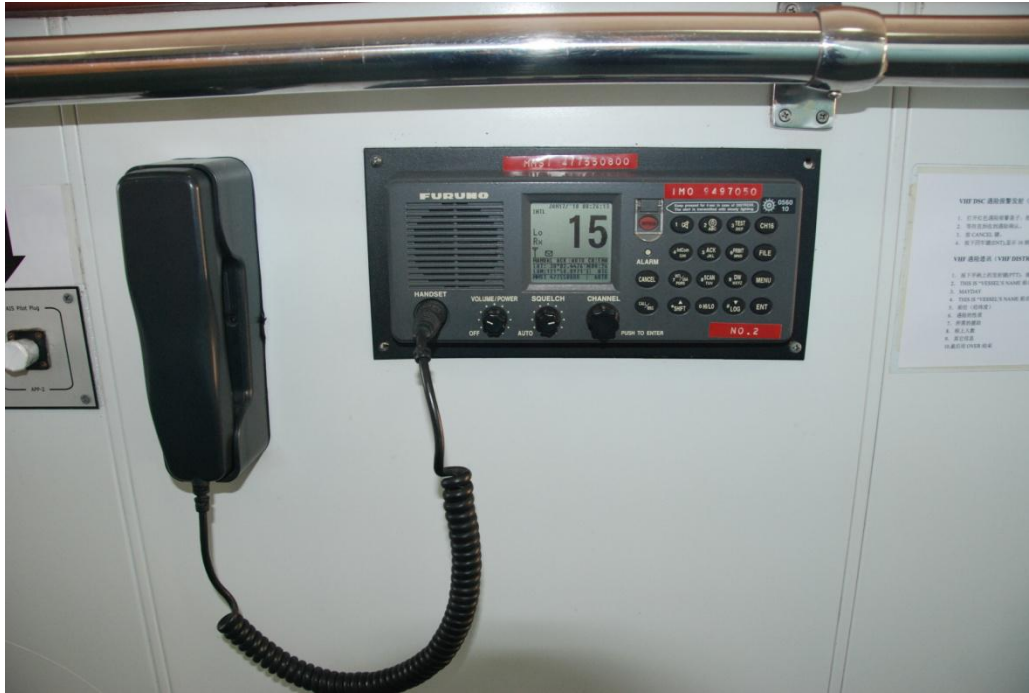
VHF (bridge front)
