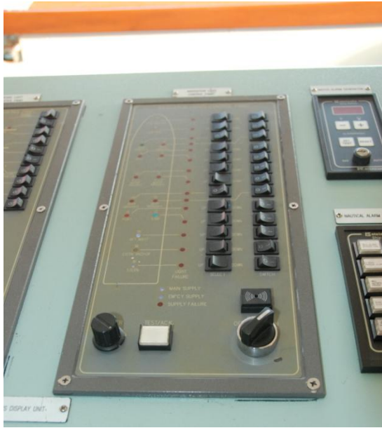
Control panel of Navigational Lights
